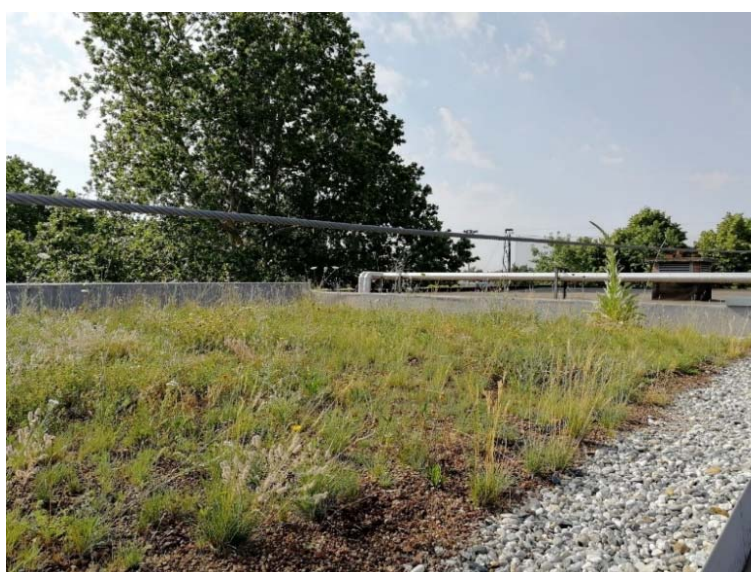
Figure 63. Overview of the Green Roof realized on the WOW building in Turin (image © City of Turin).
